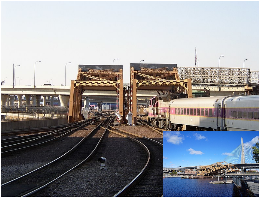
Draw 1 is a bascule type, 2-span, 4-track bridge at the mouth of North station. An MBTA commuter rail train has just departed the platforms for an outbound trip. The platforms are just 1,000 feet away. Photo: Wikimedia Commons By Lexcie, CC BY-SA 3.0. Inset: Draw 1 shown in the up position to allow boat traffic to pass through. Photo courtesy of MassDOT.
